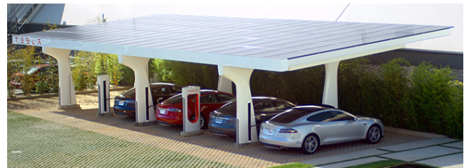
Figure 1: Tesla Supercharger equipped with PV panels [2].
